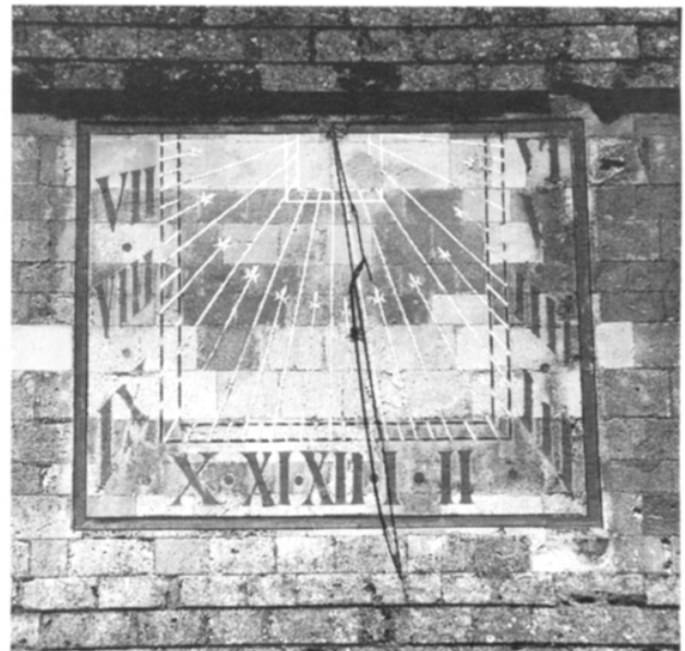
FIGURE 5: The vertical declining sundial on the southwest corner buttress of Chichester Cathedral.
