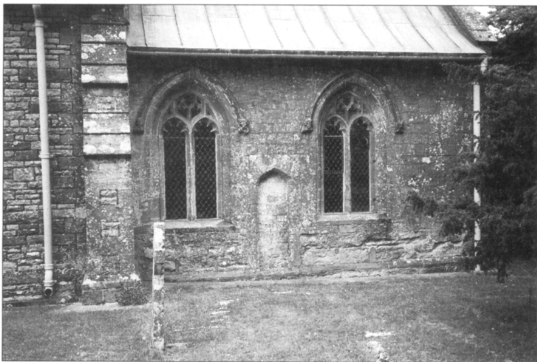
FIGURE 2: A closer view of the two windows with a blocked-up priest's door between them
